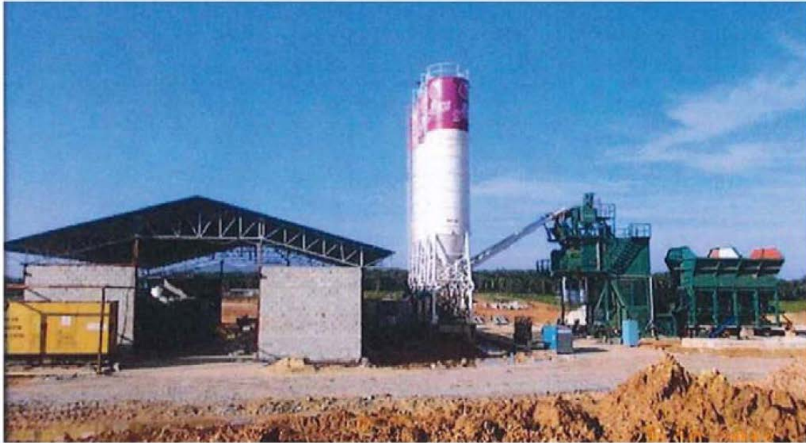
Figure 4.2-1 Batching Plant and Cement Tower Setting up at Precast Yard Area at KM. 16.5
